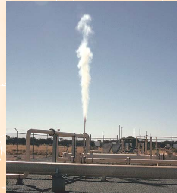
• Blowdown at Wiluna Compressor Station
